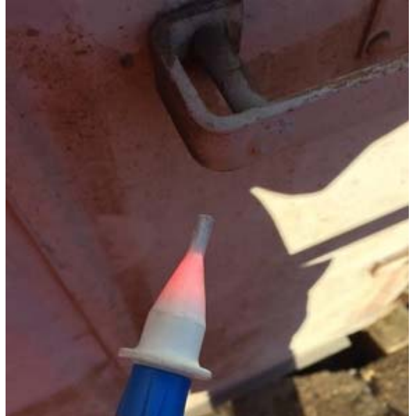
Volt-Stick showing the location cabinet is live during "Test before touch"
